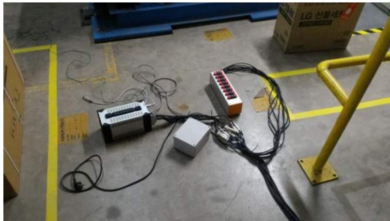
Figure 7. Strain gauge network equipment
