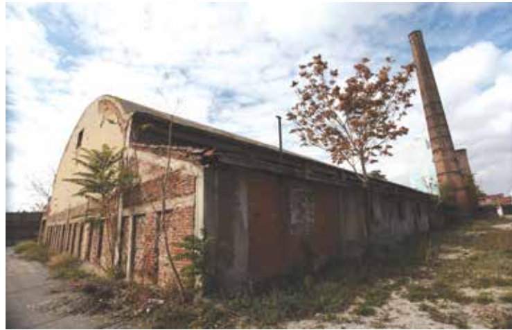
Levha 5 - Kılıçoğlu Tuğla Kiremit Fabrikası ( www.kilicoglu.com.tr ) ve Çift Kurt Kiremit Fabrikası (Eskişehir Modern Mimarlık Sergisi, Alper Elitok arşivi) / Kılıçoğlu Factory of Brick-Tile and Çift Kurt Factory of Brick (Eskişehir Modern Architecture Exhibiton; archive of Alper Elitok)
