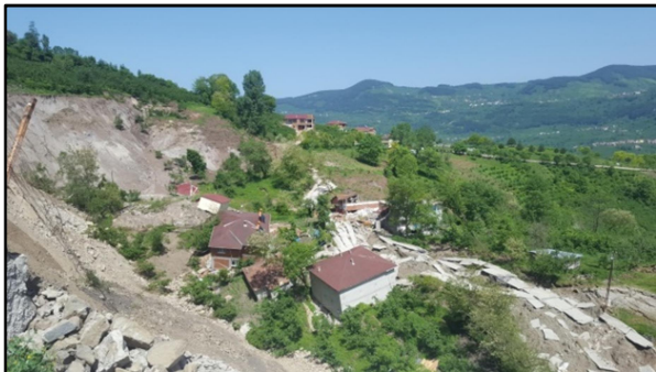
Figure 7: Some houses maintained their integrity even though their vertical status was impaired during the collapse. A view from the east.
