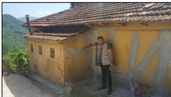
Figure 10: Some of cracked walls were repaired in 2015 but later these cracks were reopened.
