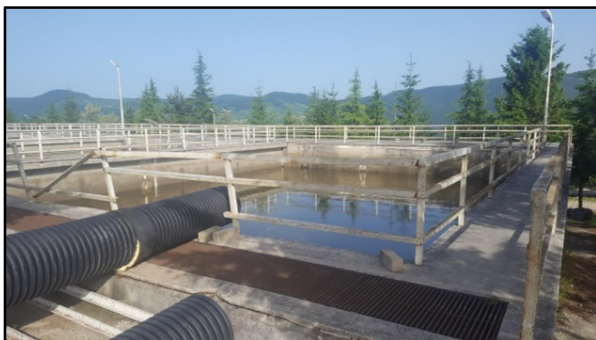
Figure 4: Aybastı Drinking Water Treatment Plant at the top of the landslide area.
