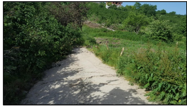
Figure 5: One of roads that cross the slope of the landslide. The road was closed to traffic after the landslide.
