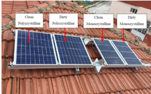
Figure 1: The views of the panels on the roof.
