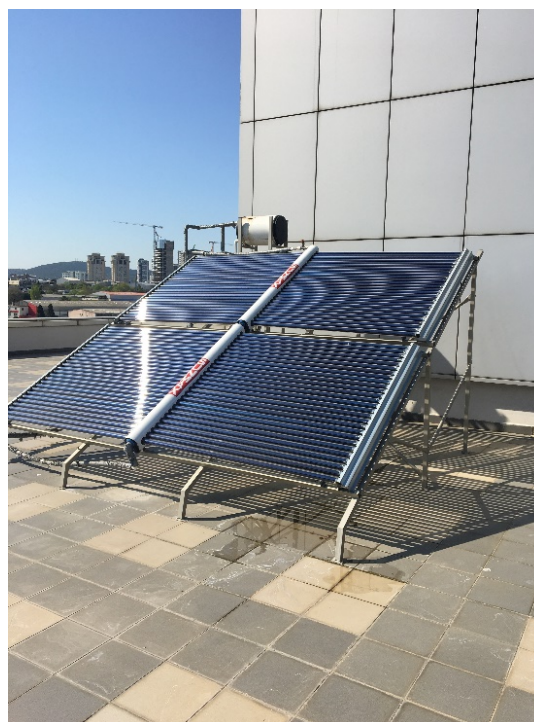
Figure 1. ETHP solar collector
