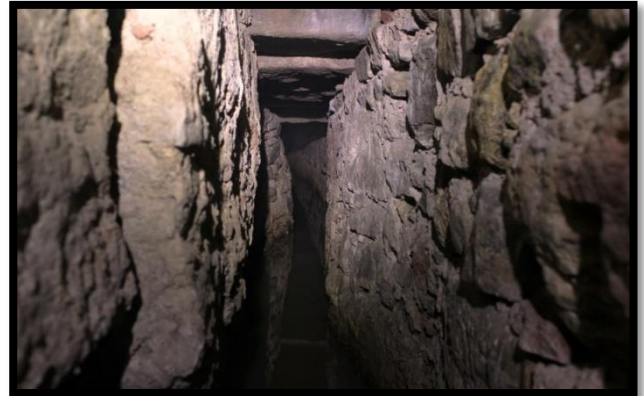
Fig. 6. Water tunnel with deformation after ground movements. The tunnel narrowed to 20 cm at some points.
