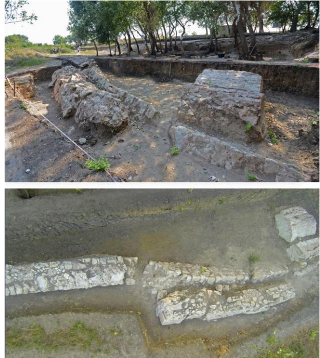
Fig. 8a-b. Laterally collapsed wall in the water structure due to probable earthquake effects.
