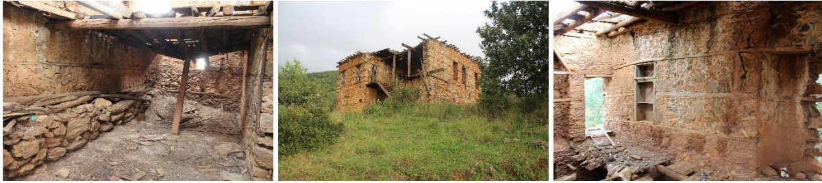
Figure 5. Ground Floor "Avla," General View of the Building, and South Wall Qibla Niches
