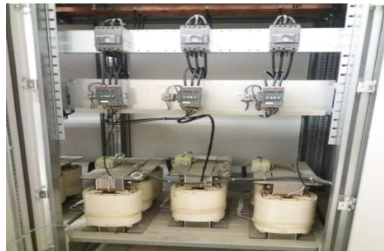
Figure 2. The shunt reactor panel.
