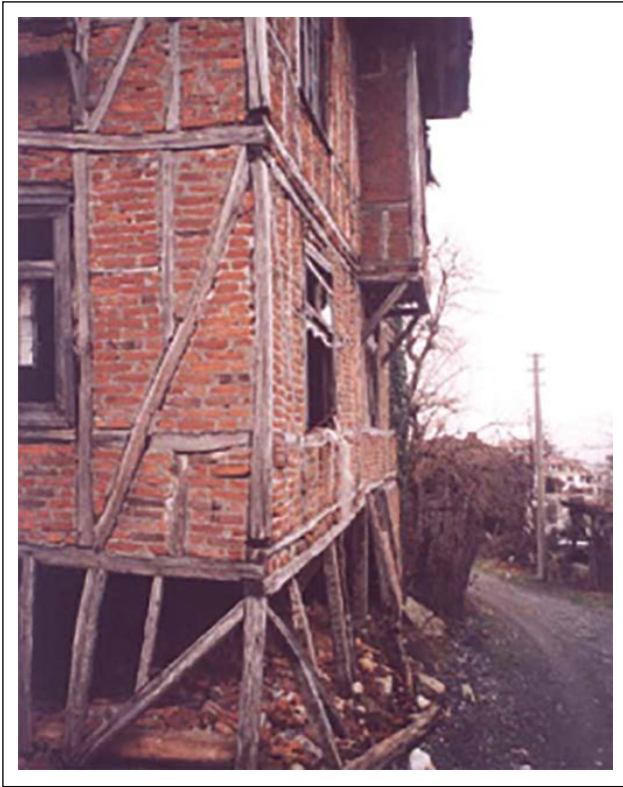
Figure 2. Soft story damage in a traditional wooden structure, 1999 Düzce earthquake [7].
