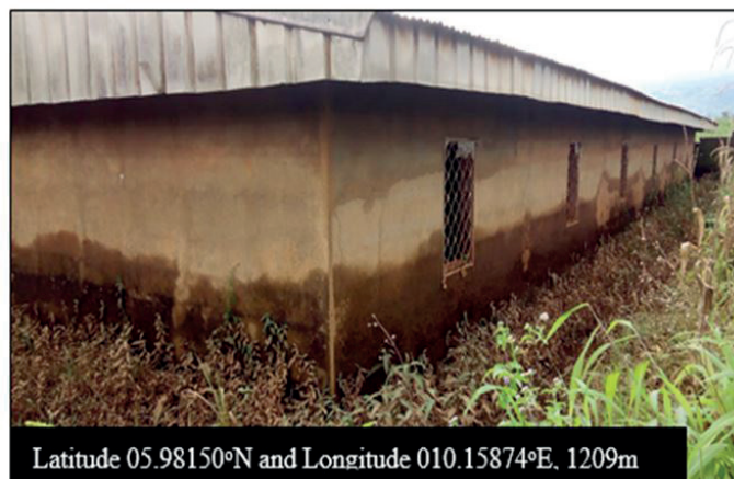
Photo 4: Abandoned structure on wetland at Mulang (Field Survey, 2020).
