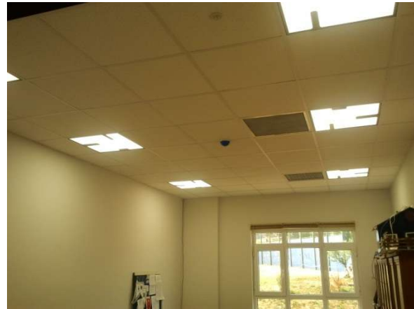
Figure 1. Test Room 1 (LED)
