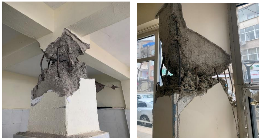
Figure 7 Column damage due to insufficient transverse reinforcement
