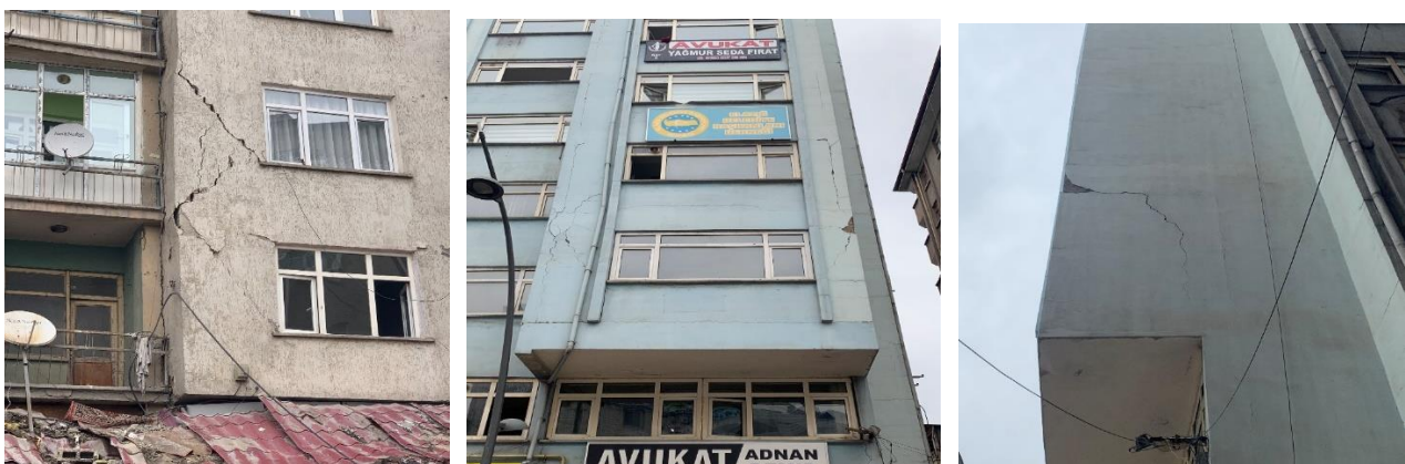
Figure 14 Damages of overhang infill walls
