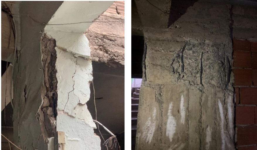
Figure 8 Buckling longitudinal reinforcement bars of damaged column due to insufficient transverse reinforcement
