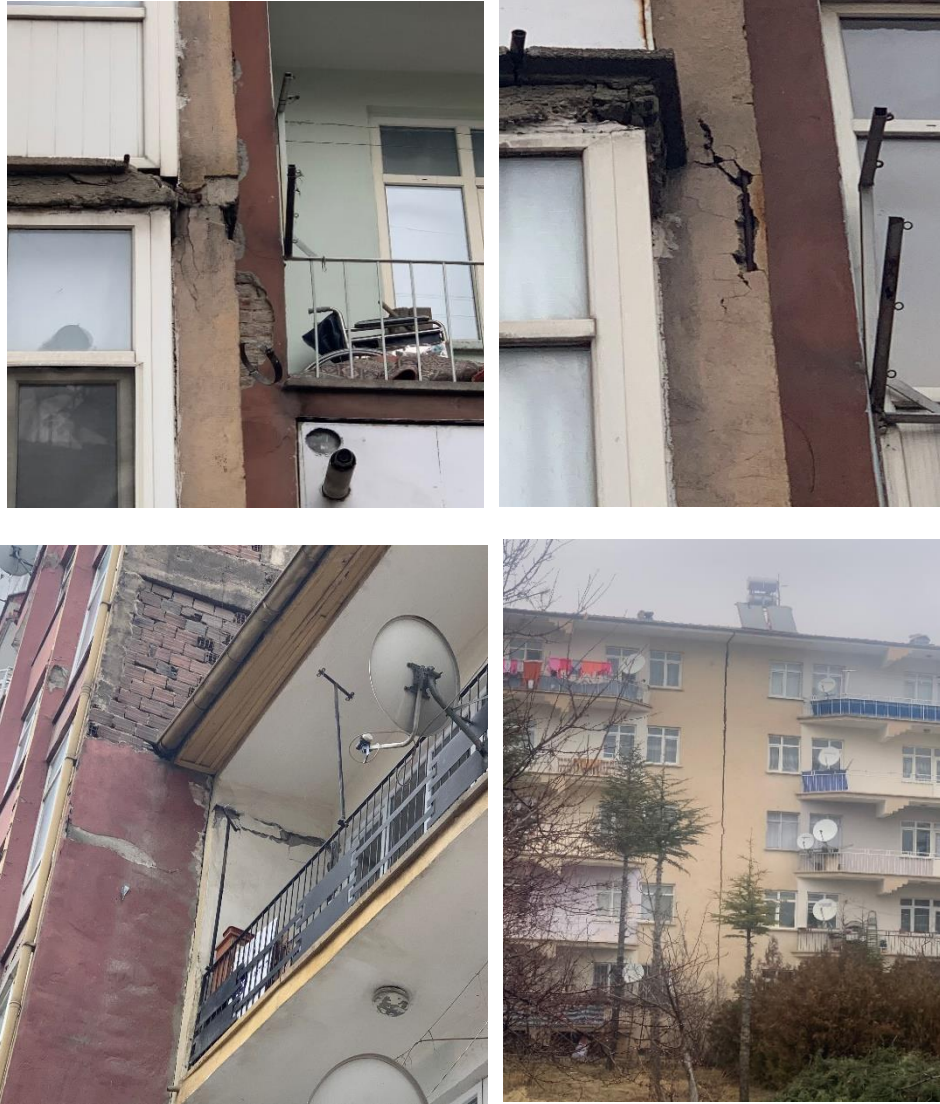
Figure 15 Damages of adjacent buildings
