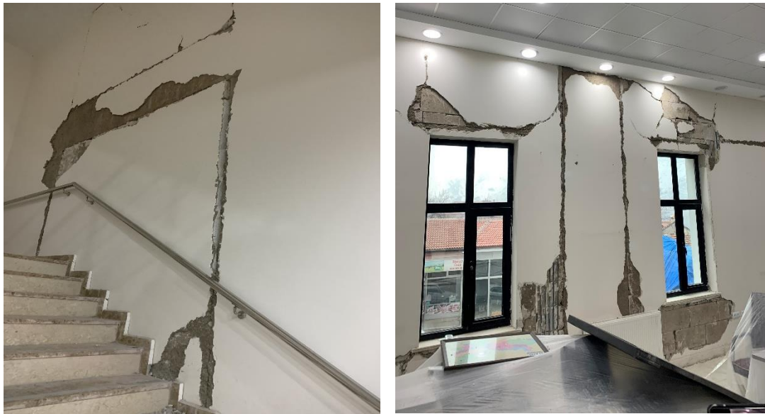
Figure 13 Disconnection of infill wall from the frame
