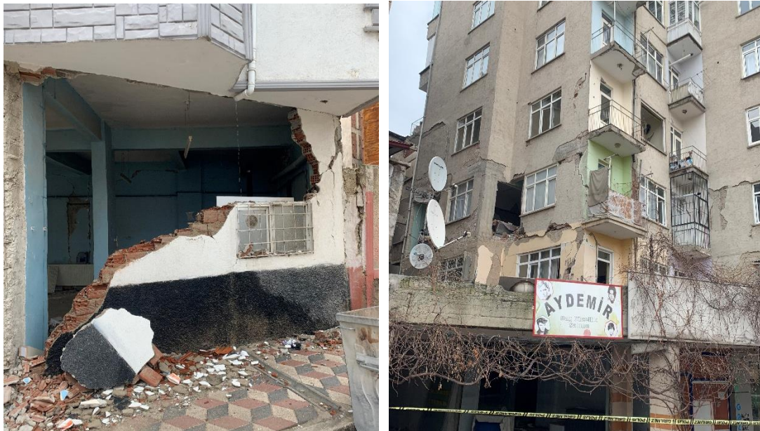
Figure 12 Partial out-of-plane damage
