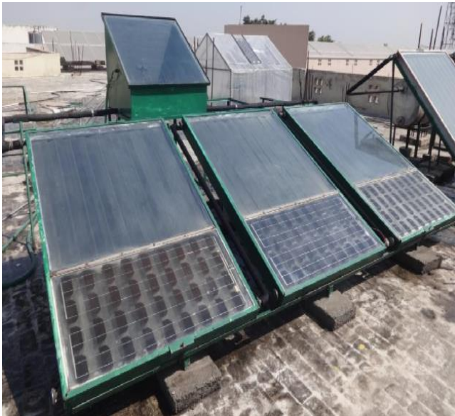
Figure 22. Photographic view of PV/T flat plate collector [79].
