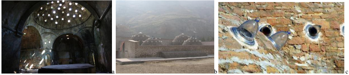
Figure 5. On The Left, the Skylights of the Historical Turkish Bath in Unye, in the Middle, and on the Right Sille Turkish Bath, Konya. The Glasses in the Bath are Made Concave to Increase the Endurance to High Temperatures. a-(URL 3) b- (URL 4) c- (URL 5)
