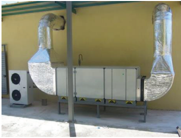
(b) air conditioning
