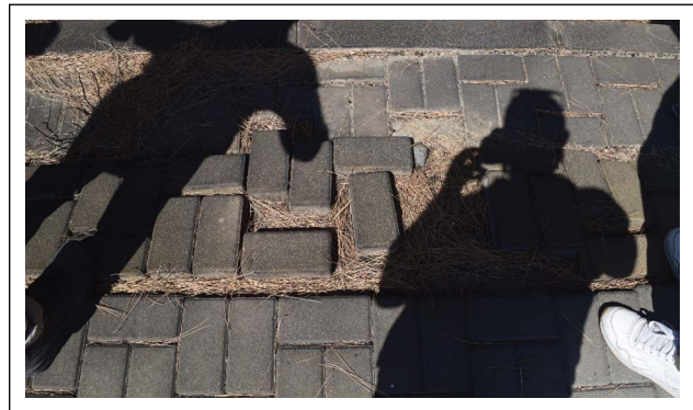
Figure 2. Pavement in the fire zone.
