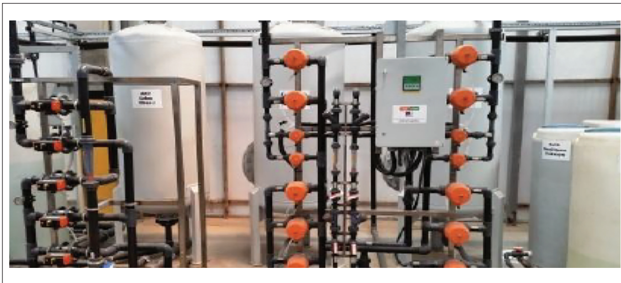
Figure 2. Demineralisation unit in Facility-A.
