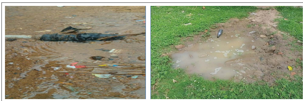
Figure 2. Broken pipes indicating potential contamination pathways within the city.
