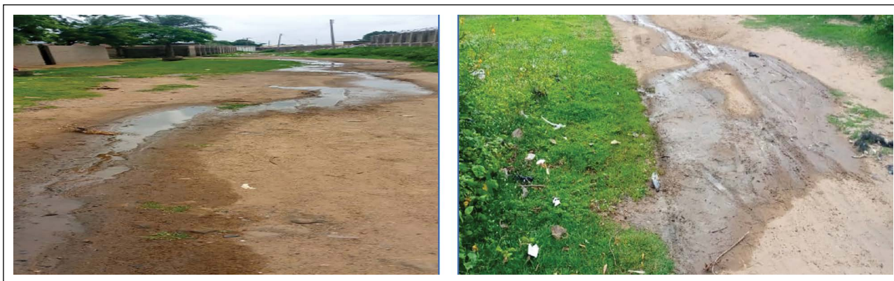
Figure 5. Water loss during pumping due to broken pipes within the city.
