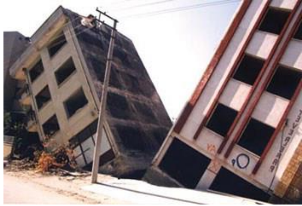
Şekil 4. Devrilen bina No:2 (H=10,00 m, B=5,00 m), (H/B=2,00) [24] (Overturned building No:2 (H=10,00 m, B=5,00 m), (H/B=2,00) [24])
