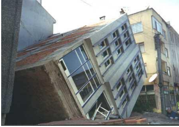
Şekil 3. Devrilen bina No:1 (H=13,50 m, B=7,50 m), (H/B=1,80) [24] (Overturned building No:1 (H=13,5 m, B=7,50 m), (H/B=1,80) [24])
