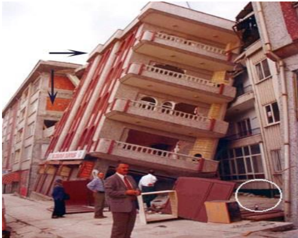
Şekil 5. Devrilen bina No:3 (H=13,50 m, B=6,50 m), (H/B=2,10) [24] (Overturned building No:3 (H=13,50 m, B=6,50 m), (H/B=2,10) [24])
