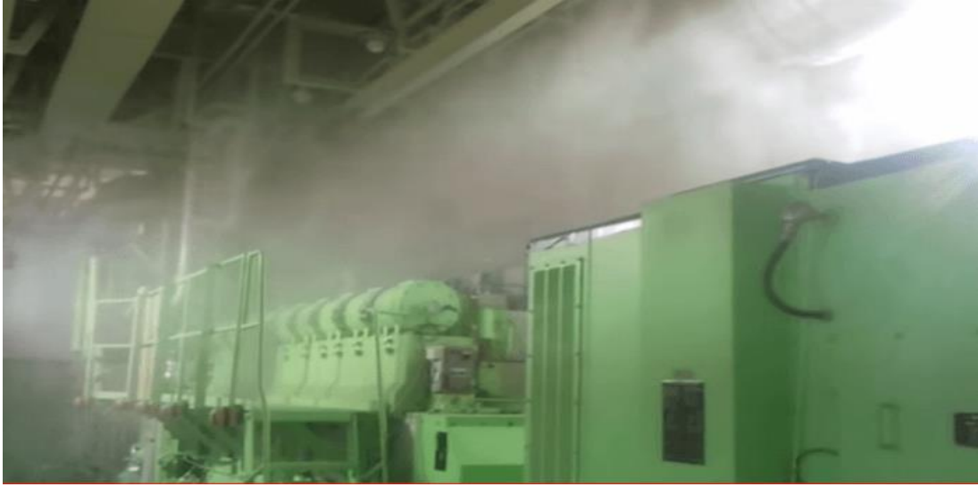
Figure 1. Water protection in Engine Room.
