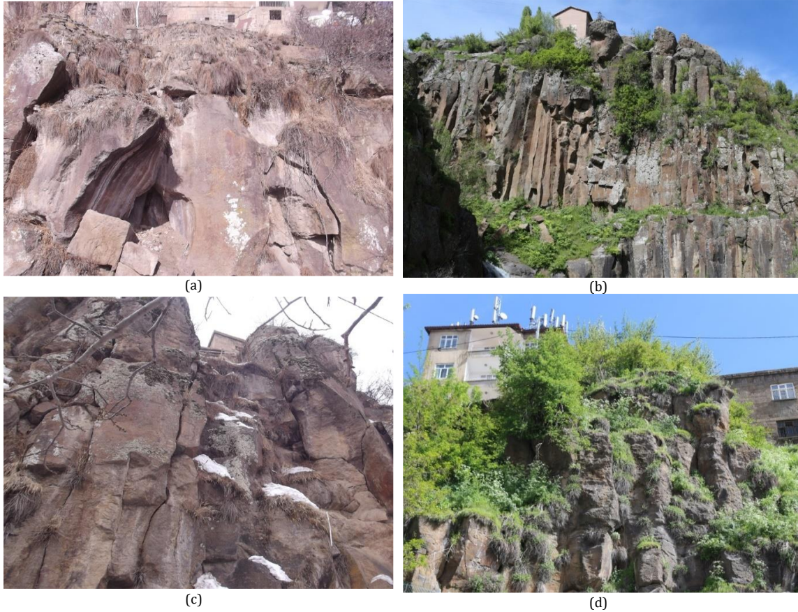
Fig. 7. Some photos of different lithological structures at risk of rockfall in the study area (a) and (b) cracked and decomposed ignimbrites, (c) Basalt columns, (d) prismatic ignimbrites
