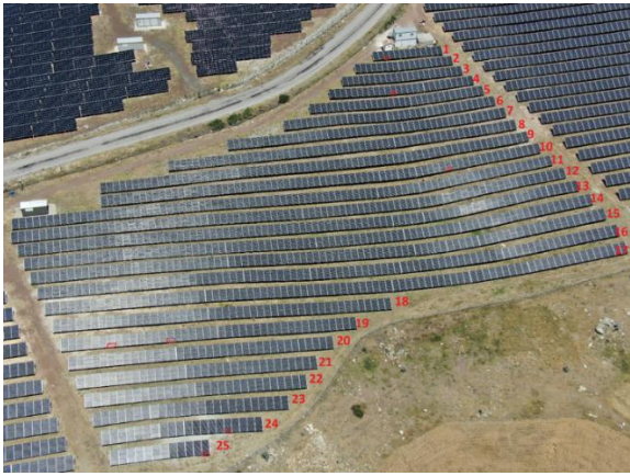
Fig. 3 2.7 MW solar power plant captured by drone
