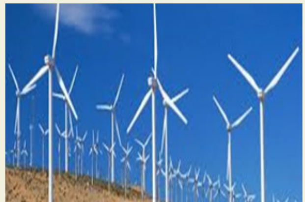
Figure 1. A photo of Wind power plant
