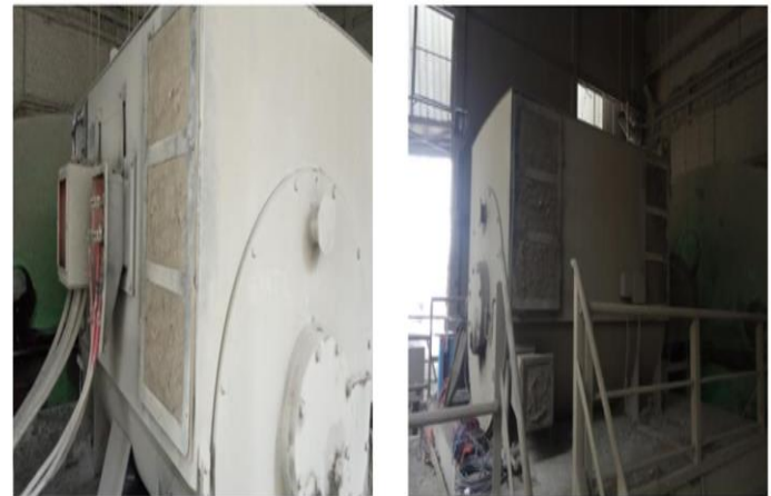
Figure 7. Cement Mill-3 Main Drive Motor General Field View
