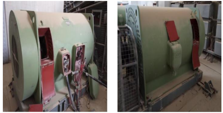
Figure 3. Crusher-1 Main Drive Motor General Field View
