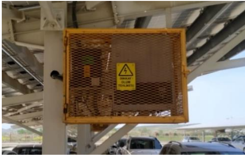
Figure 4. Inverters placed in steel cages under PV panels.
