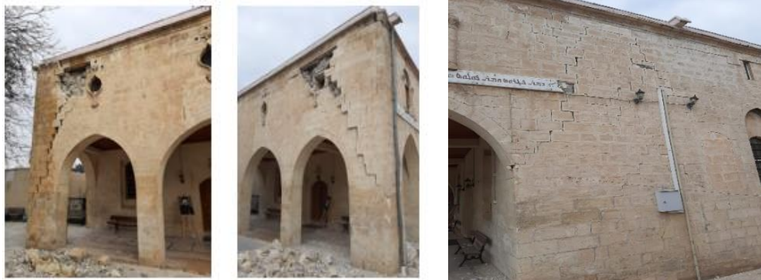
Figure 5. Shear cracks in the facade wall (2e)
