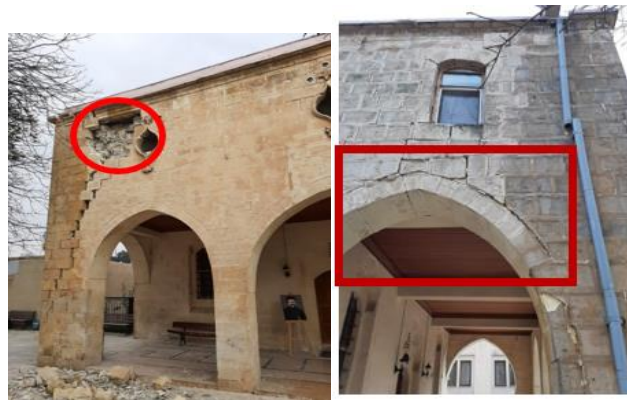
Figure 12. Damage caused by flaking or loss of parts (2a) in the element; particularly resulting from past insufficient reinforcement interventions or weakening of material strength due to lack of maintenance, and occurred during the earthquake
