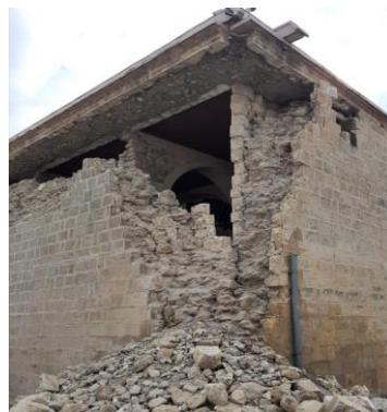
Figure 4. The damage observed between perpendicular walls due to the use of different materials or inadequate connections (2c)
