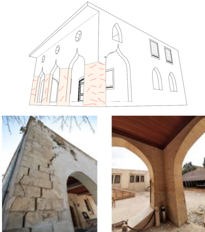
Figure 8. In the column bases, in-plane torsion or shear cracks (3b) are observed
