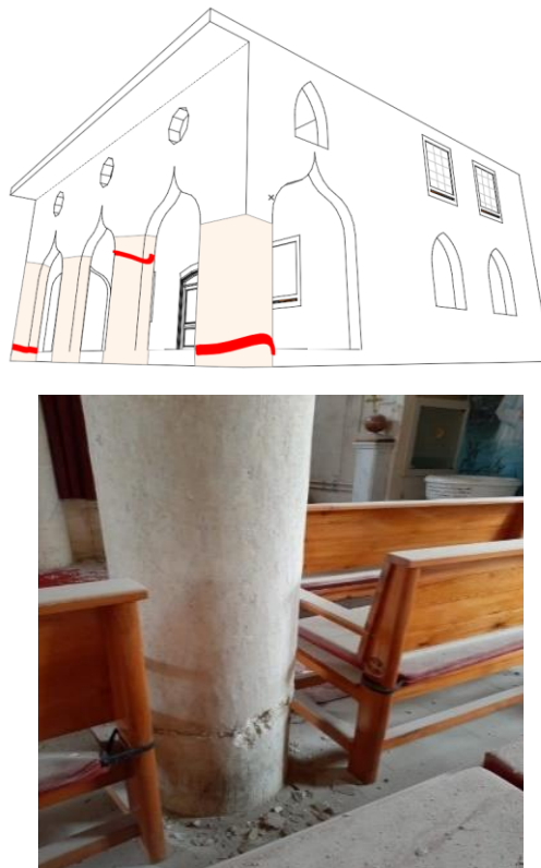
Figure 7. In the column bases, in-plane sliding cracks (3a) are observed
