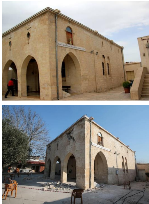
Figure 1. Adiyaman Mor Petrus and Mor Paul Church before (left) and after (right) earthquake (Karataş photo album, 2023)
