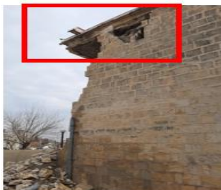
Figure 11. Damage caused by the roof at wall corners or on top of the wall (6a); Shear damage between the roof and the walls (6b), particularly due to inadequate reinforcement interventions in the past or lack of maintenance
