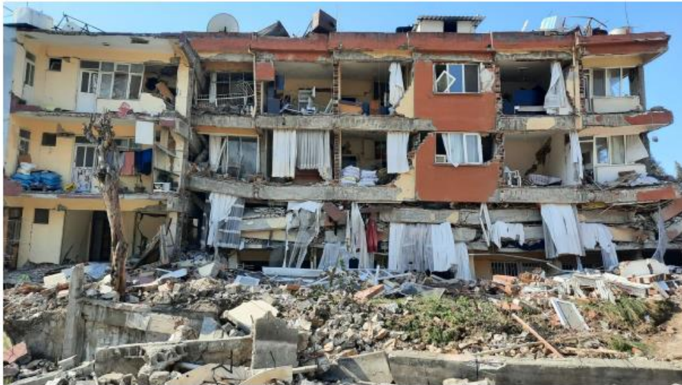
Figure 8. Hatay – city center heavily damaged and destroyed buildings (TMOBB, 2023)
