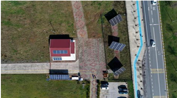
Figure 1. Solar power plant
