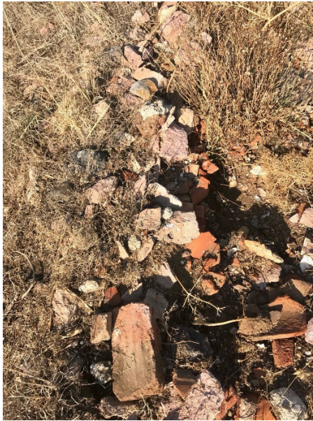
Figures 25–26. Masonry foundations and mixed debris of a collapsed building on Kumru Island, supposedly the chapel dedicated to St. George of Chios (Adramytteion Researches, 2018).
