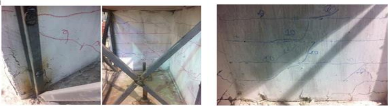
(b) Cracks on first-story shear walls
