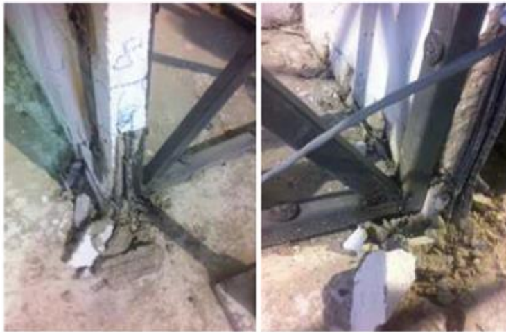
(c) Damage at wall and steel brace connections at the foundation level
