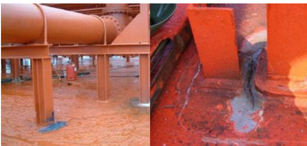
Figure 15. Cracks on pipe supports on hull main deck [6].
