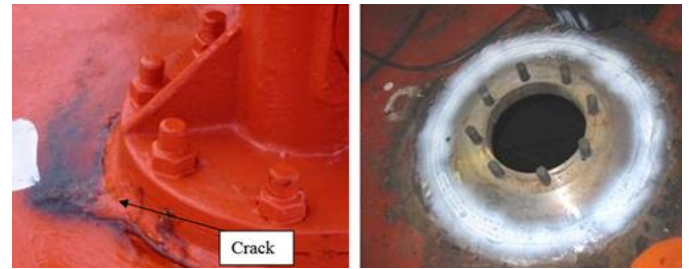
Figure 6. Crack in way of pipe penetration in main deck [3].
