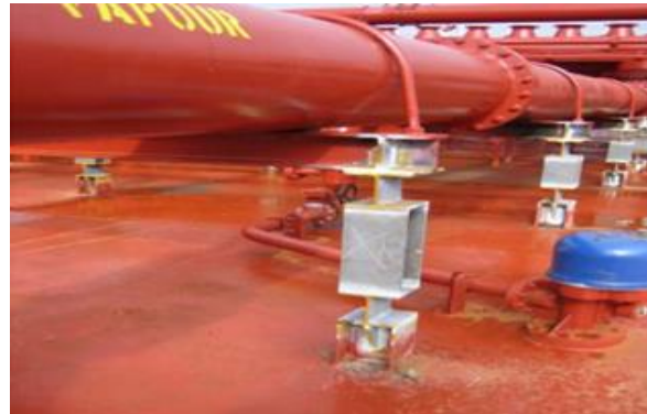
Figure 17. The flexible pipe supports.
