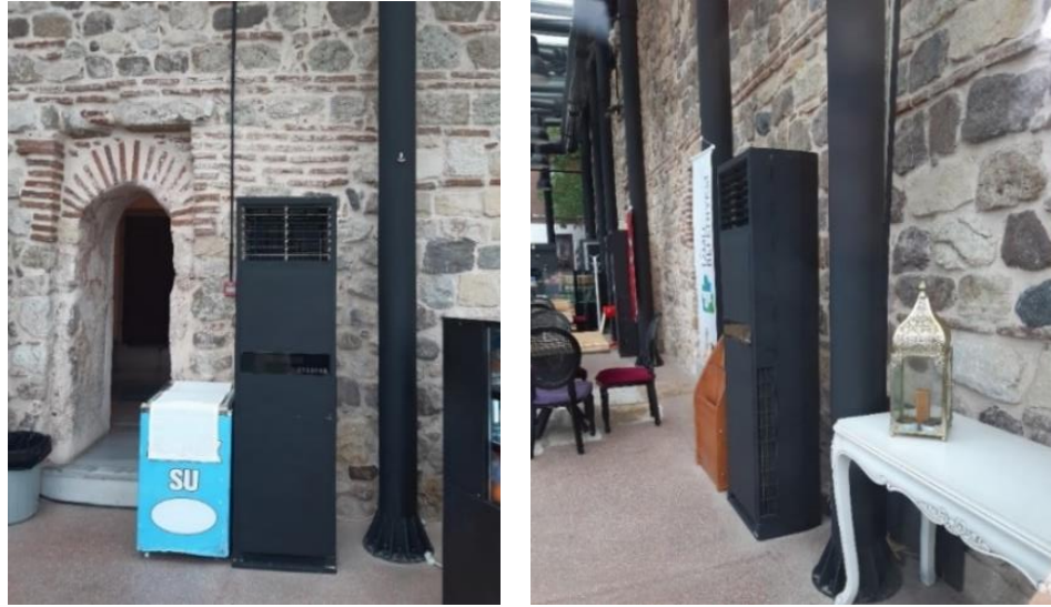
Figure 7. HVAC systems used in the restaurant of Süleyman Pasha Hamam (Personal Archive)
