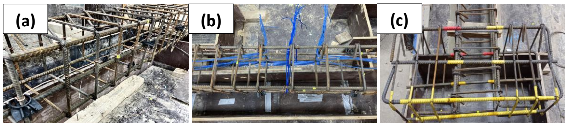
Figure 2. Copper wires used for reinforcement bars (a) Copper wires for longitudinal bars (b) Copper wires used for stirrups, (c) insulation for foundation
