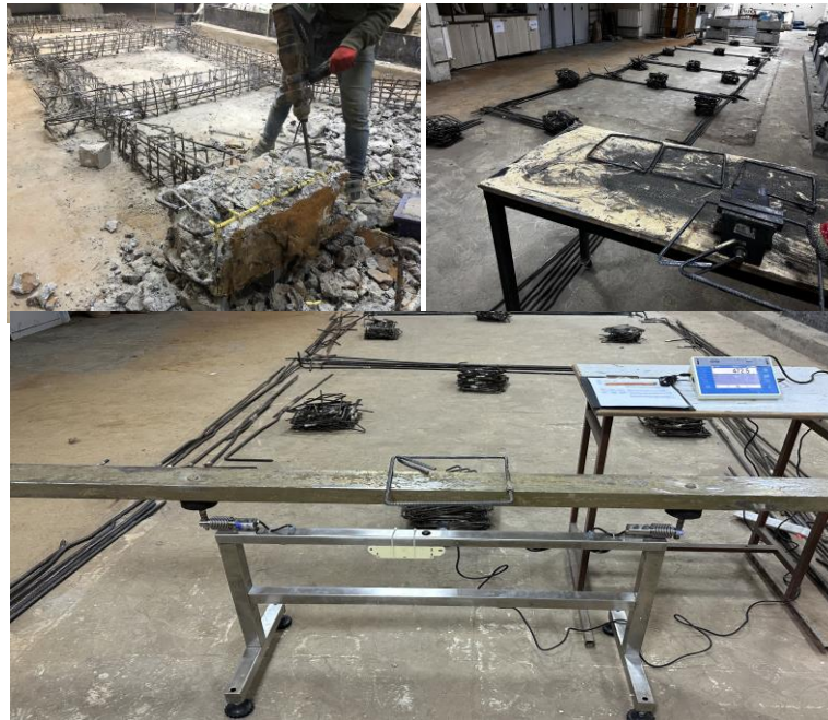
Figure 8. Acquire actual corrosion ratio (a) breaking of concrete (b) chemical cleaning (c) weighing of the all reinforcement bars
