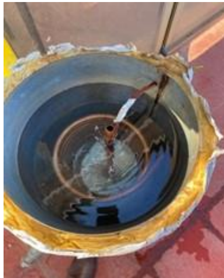
Figure 4. Hot water storage tank
