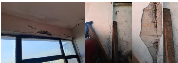
Figure 1. Reinforced concrete elements subjected to corrosion effect.
