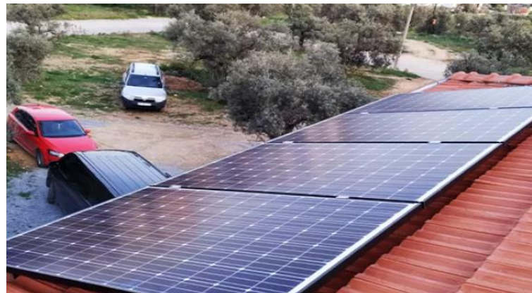
Figure 12. Excel PV-T Hybrid solar panels (Solimpeks, 2023).
