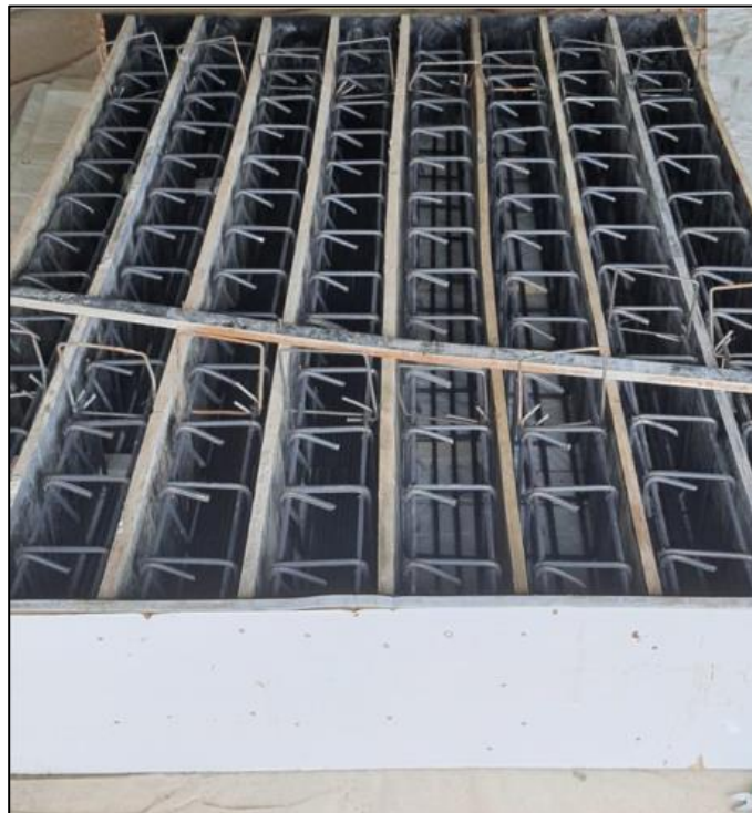
Figure 2. Preparation of reinforcement of beam specimens and placing them in the mould.
