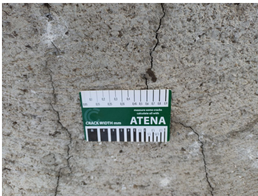
Fig. 5. Cracks observed at deck top surface
