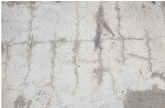
Fig. 7. Plastic settlement cracks
