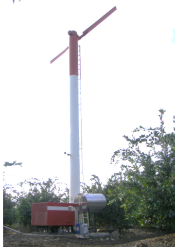
Figure 1. General view of wind machine
