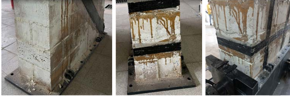
Fig. 14 - Observed crushing failure in toe regions of the walls.
