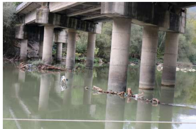
Photo 6. Low water level under Filyos V Bridge (October 2015)
