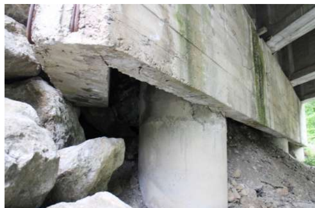
Photo 7. Abutment of Filyos V and settlement at bridge approach filling
