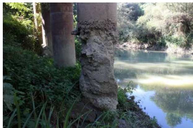
Photo 3. Abrasion on pier of Bartın I Bridge
