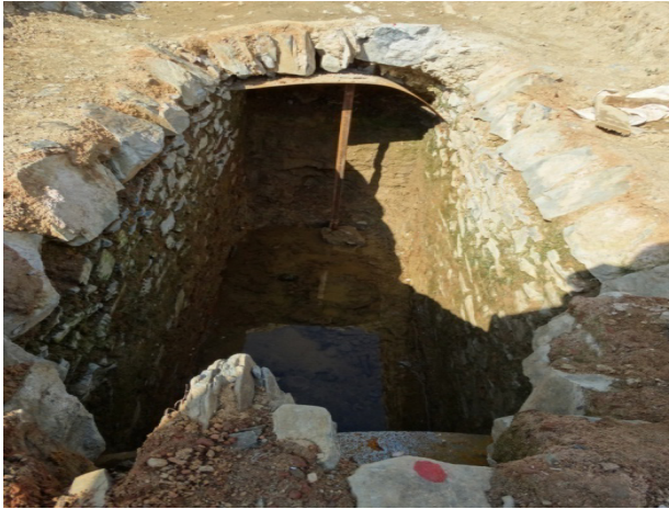
Figure 7: Damaged vault from the original phase of the aqueduct channel.
