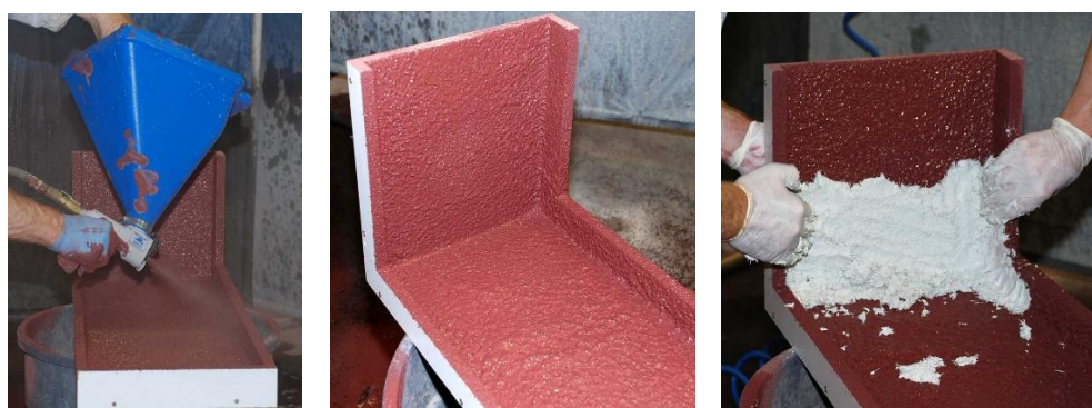
Figure 4. Spraying the face coat-face coat ready for backer mix-hand packing backer on upright [11].
