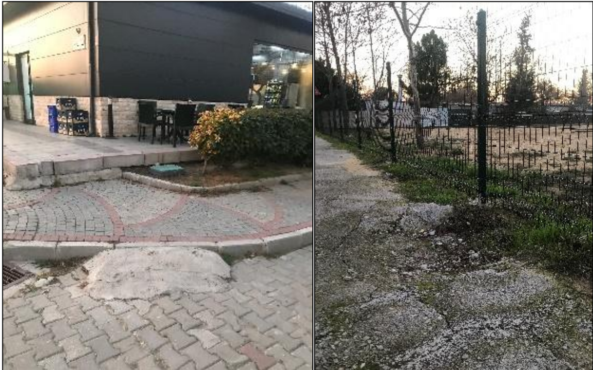
Figure 3. a) Pavements and curb ramps near the Kepez Public Cafe and b) Deteriorations in the pavement materials (Original, 2023)
