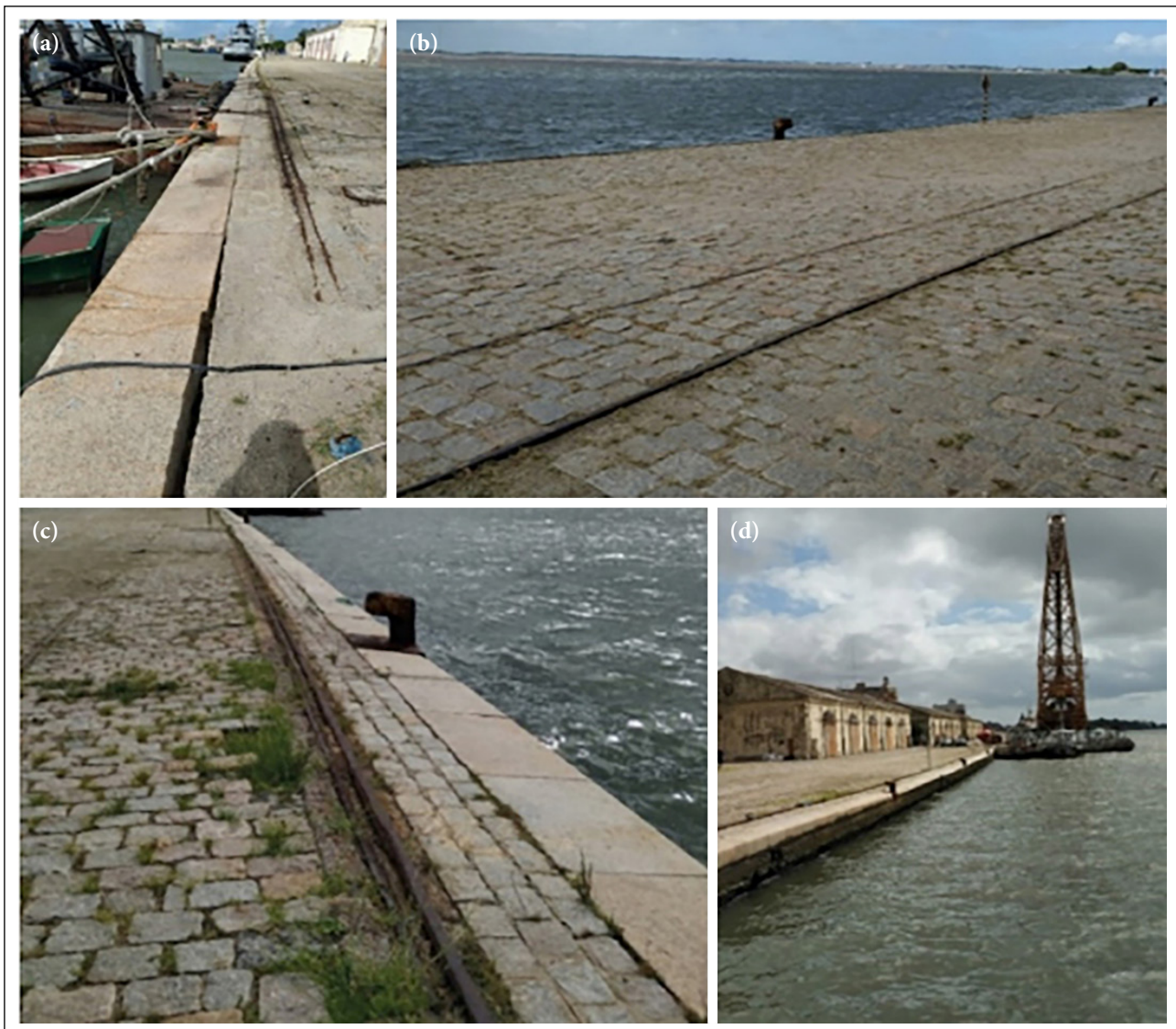
Figure 2. (a) Displacement of the pier structure blocks. (b) Height variation along the pavement and pier crown blocks. (c) Displacement of the gravity wall towards the navigation channel. (d) Area where displacements are most intense.
