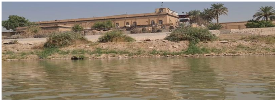
Figure 12. Neglect of the riverbank adjacent to the Ministry of Defense and the Abbasid Palace / Source: Field visit
