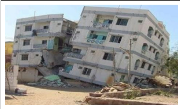
Figure 1. Soft storey building failure during Gujarat Earthquake (2001) in India [1].
