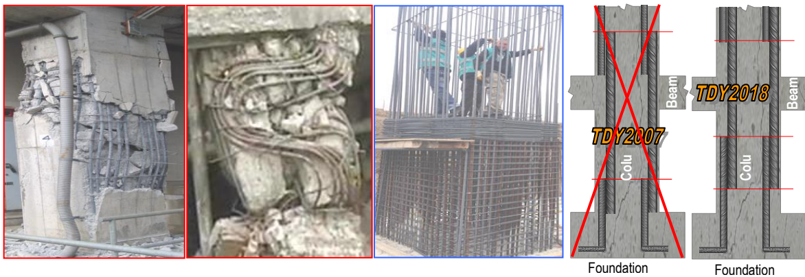
Figure 2. Damages of reinforced concrete columns and effect of reinforcement arrangements
