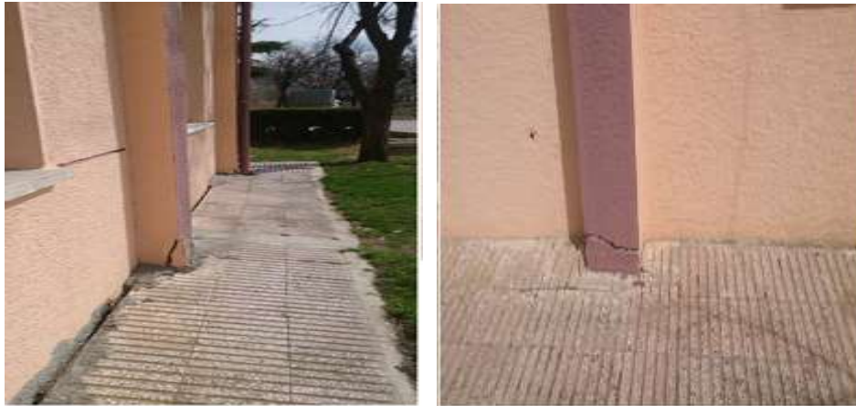
Figure 7. The deformations observed in the study area after detonations
