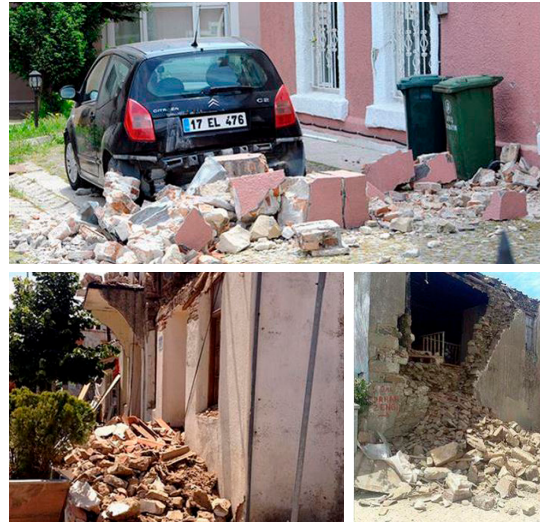
Figure 17. Some examples of heavily damaged house from Gökçeada Island and Çanakkale (Turkey; by AA).
